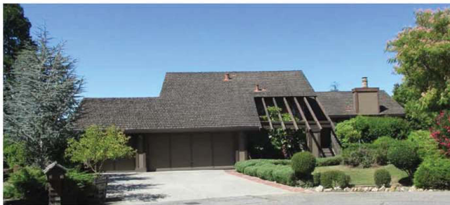
Photo 5. Combustible Wood Roof.
