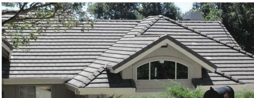
Photo 26. Noncombustible roof covering. Leaf litter removed.
