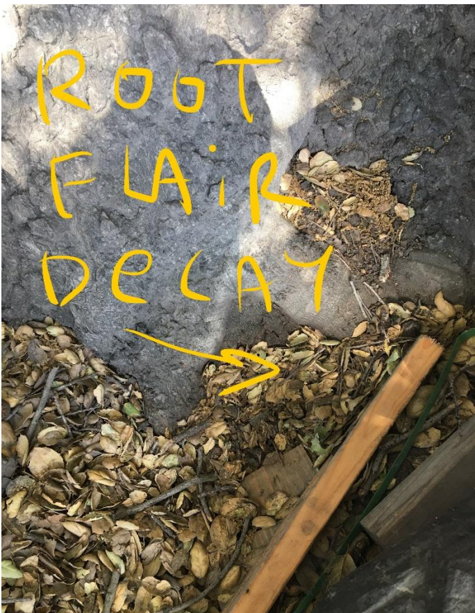
#11955- Root flare decay
