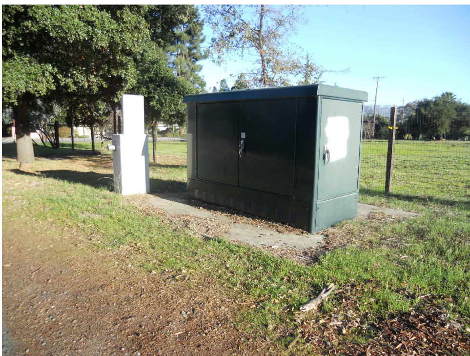
UTILITY VAULTS NEAR THE SABINI INTERSECTION WITH TERESA LANE.
