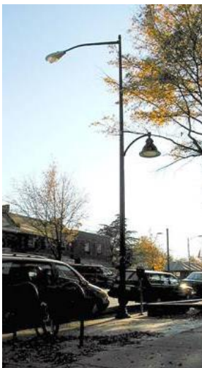
Figure 2-18: Traditional design of a combined roadway and pedestrian-scale light fixture
