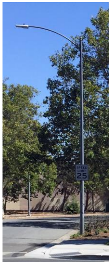
Figure 2-15: Roadway cobra head light fixture
