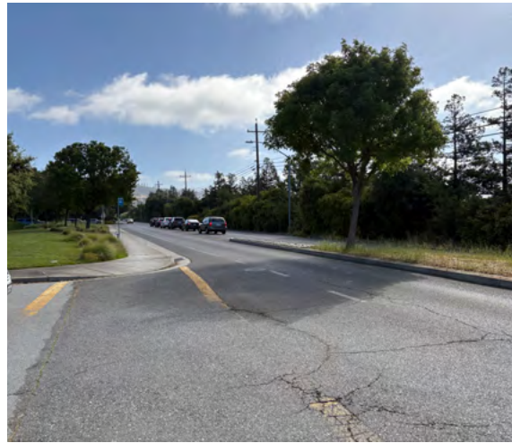
FIGURE 22 Faded crosswalk at Ann Sobrato High School
