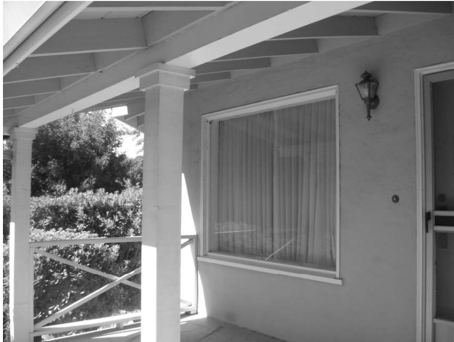
Photo 5: View of the porch showing exposed rafters.
