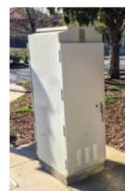
Example of Main Box in Morgan Hill
