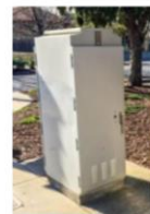
Example of Main Box in Morgan Hill
